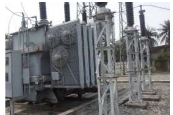
Transformers installation for Al Iraquia satellite channel, Baghdad
