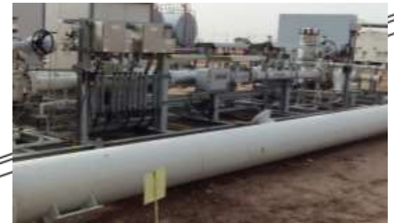
Installing KROHNE Custody transfer metering system in the off-loadings Station for Kuwait Energy Company
